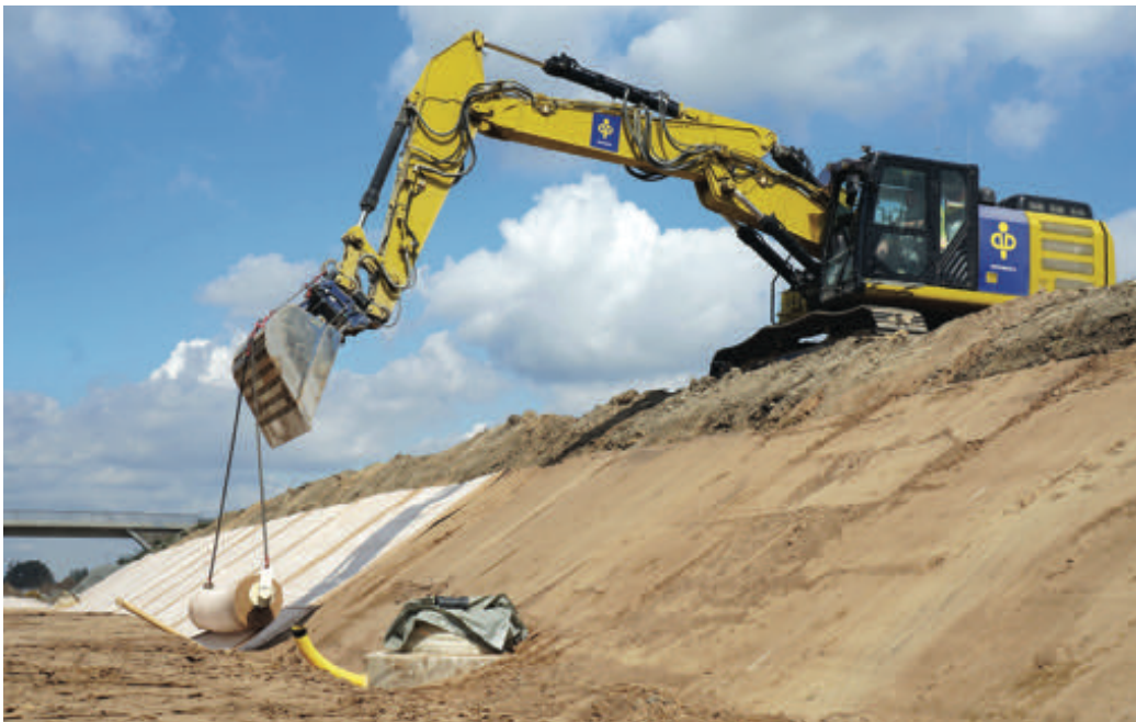
Figure 7 – Use of a bentonite mat to protect groundwater on the A33 motorway, Halle, Germany.
