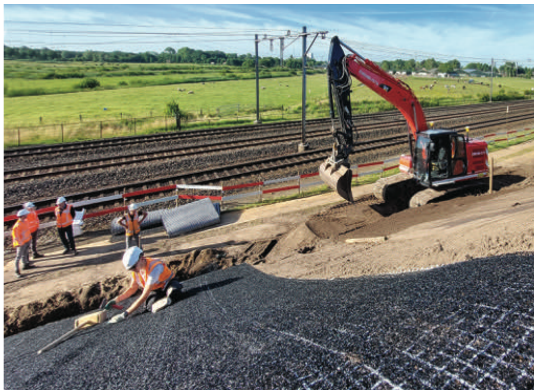
Figure 9 – Installation of a permanently reinforced erosion control system, securing an embankment slope next to a railway, Groenekan, The Netherlands.
