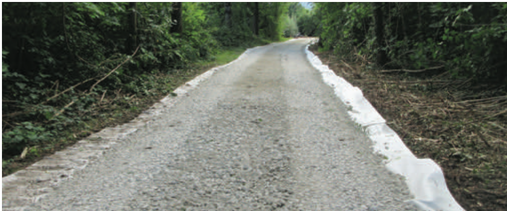
Figure 10 – Biodegradable nonwoven made from renewable raw materials as a separation and filter layer in a temporary construction road, Dettingen, Germany.
