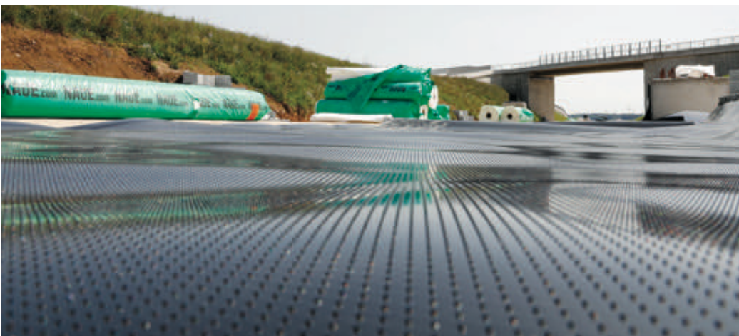
Figure 8 – Sealing the subsoil for groundwater protection with a HDPE geomembrane and nonwoven protection layers at the railway Wendlingen-Ulm parallel to the A8 federal highway, Germany.
