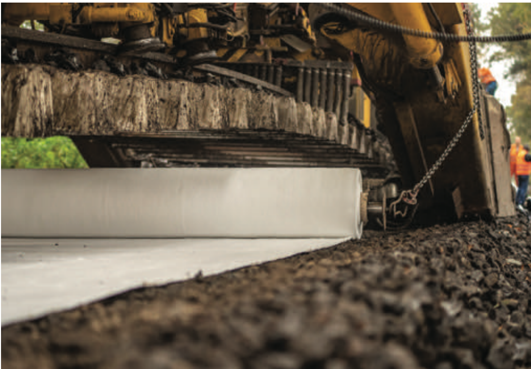
Figure 4 – Separating geotextile between the fine-grained subgrade and the coarse-grained base course layer in railway construction.
