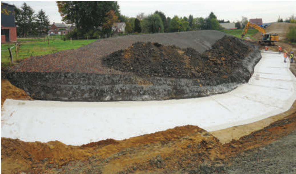
Figure 2 – Dyke foreland improvement with a bentonite mat creating sufficient length against the piping phenomena and meeting the Limburg Water Board design requirements for flood defence, Neer, The Netherlands.
