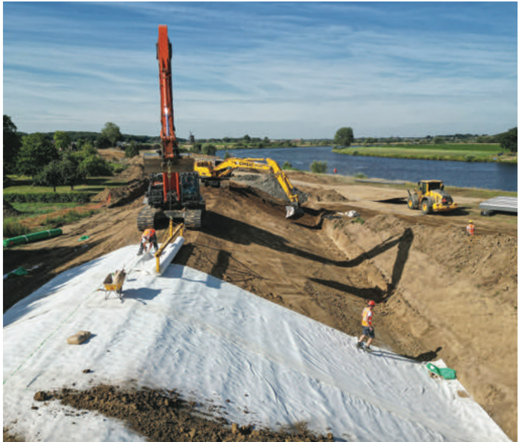
Figure 3 – Dyke improvement with installation of a bentonite mat on the crests and slopes of the flood defence to replace a full clay cover of 1 meter and stimulating re-use of local soil, Beesel, The Netherlands.
